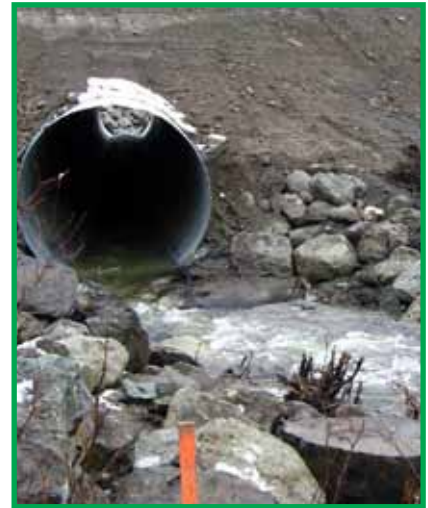
Closed bottom culvert. The culvert must be angled to allow water to flow freely through the culvert.
