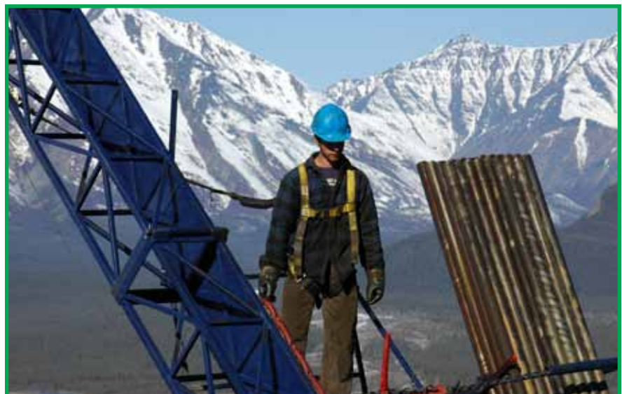
Contracts with contractors should stipulate that employees wear proper PPE for the job.
