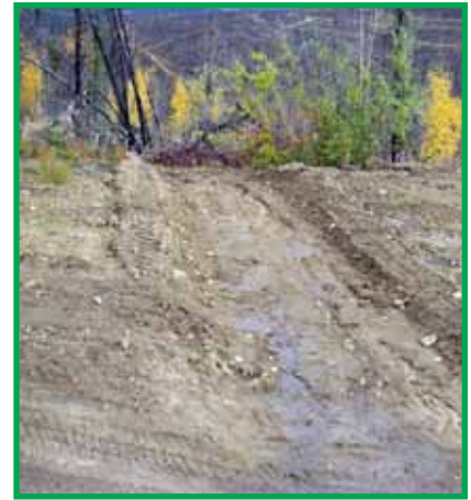
Water bar in action. Note surface water is diverted from flowing down the road surface.
