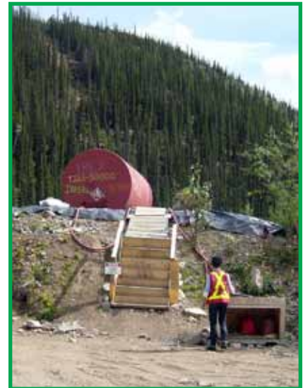
Stationary fuel containers with secondary containment. Note earth berm lined with plastic and signage posted at foot of stairs and on the fuel tanks.
