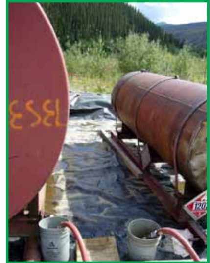
Close up of the secondary containment. Note the earth berm is lined with plastic, fuel nozzles placed in buckets to collect drips and signage is posted on the fuel tank.
