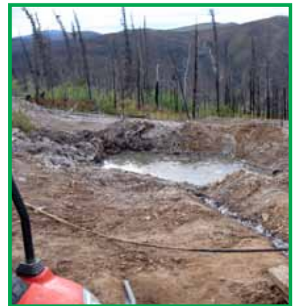
Sumps can be used to collect drill water. After the drill program is completed all sumps must be filled in.
