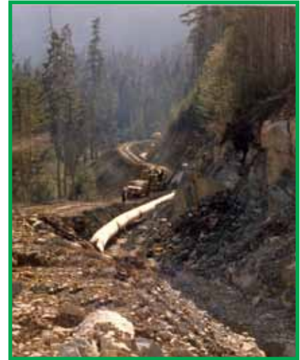
Ditches and culverts should be designed not to discharge water directly into watercourses or onto erosion prone slopes. Note the ditch is “u” shaped.
