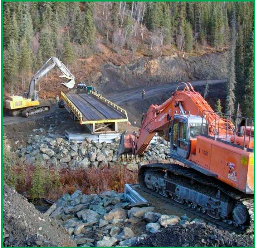
Equipment for this construction project is operated from above the stream bank. Note erosion control measures, silt fences lower left, in riparian zone.
