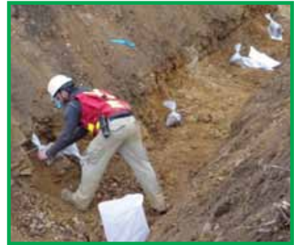
The sides of trenches should be sloped to a stable, safe angle to limit the safety risk associated with entrapment from slumping.
