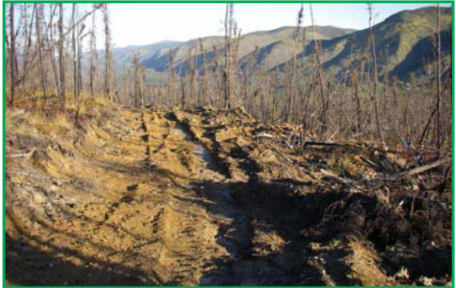
If rutting and gouging occurs the disturbed area must be restored by re-grading and draining the surface water away from the road.
