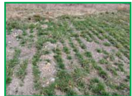
Scarified soil with vegetation growing in the grooves made by the bucket.
