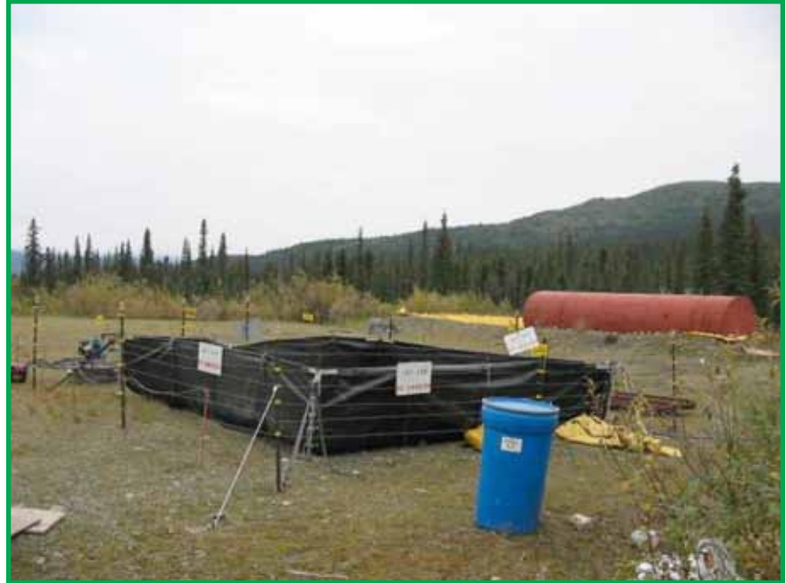
Photo showing two different types of fuel storage systems. In the foreground a fuel bladder is stored within a portable berm surrounded by an electric fence. Note signage and spill kit (blue container). In the background a stationary fuel tank is placed in an earth berm lined with plastic. Note: proper storage and handling of fuel will reduce the potential effect of spills and the cost of site reclamation.
