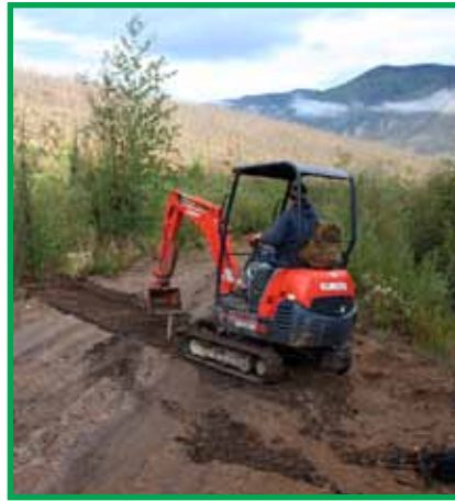
Construction of a water bar to divert surface runoff. Water bars should be constructed at an angle and in the fall to help divert spring runoff.
