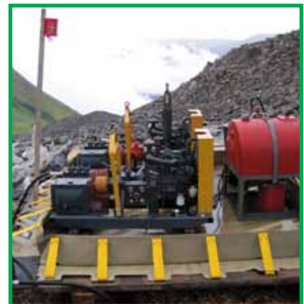
Mechanical equipment placed in an impermeable liner resistant to the product being used to collect drips and spills.
