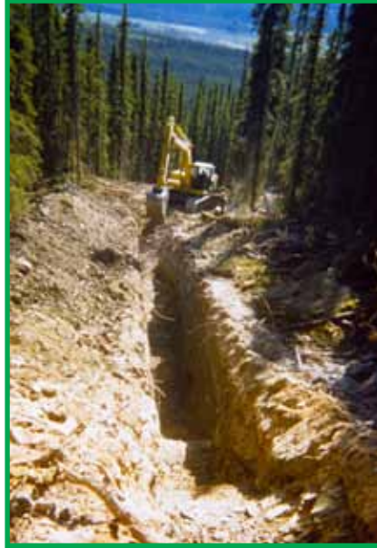
Trench dug using a back hoe. Note top soil and substrate material should be piled a safe distance to the side of the trench.
