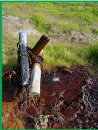
Drill hole making water before being capped.
